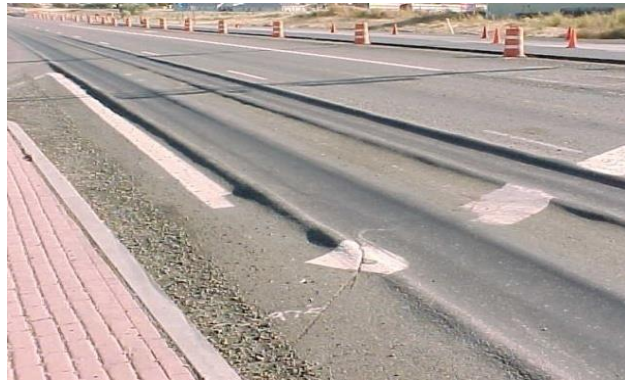
Figure 4: Rutting mode of failure
