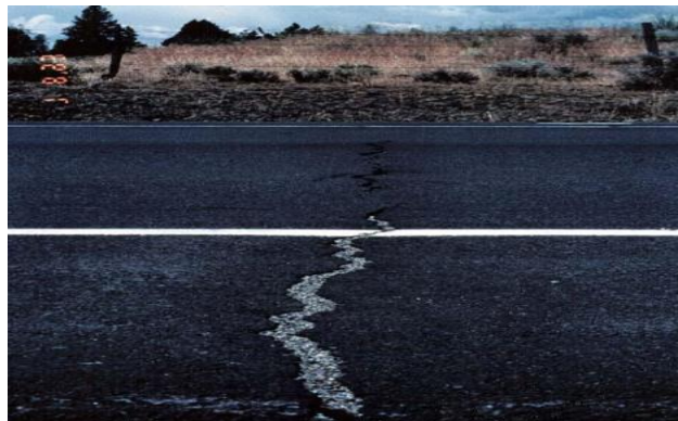
Figure 3: Low temperature cracking mode of failure
